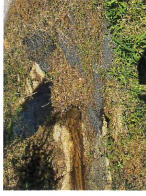
IMG_407-View Upstream Drain Clogged with Debris
